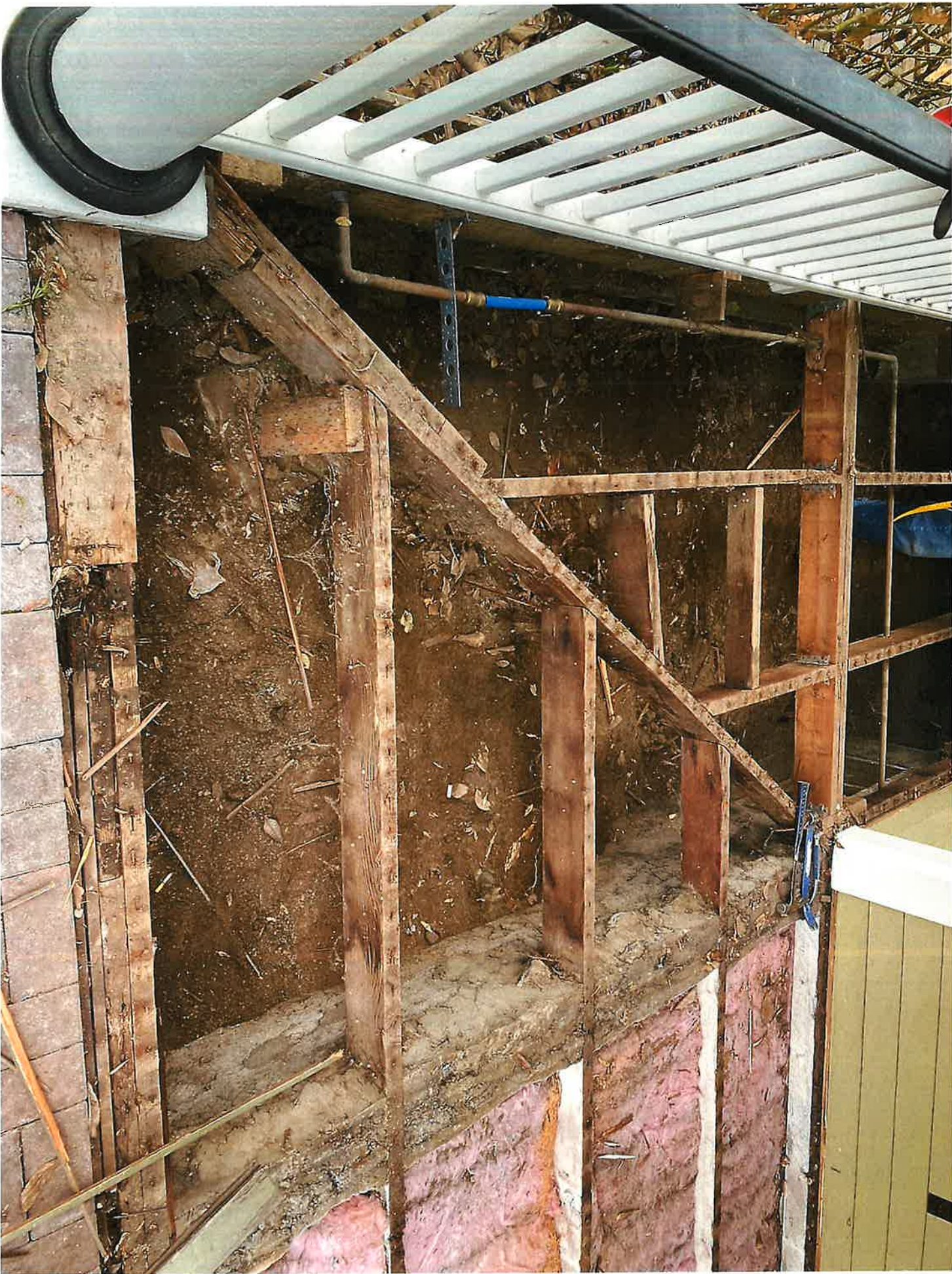
Rear porch - rot damage - needing to be replaced
