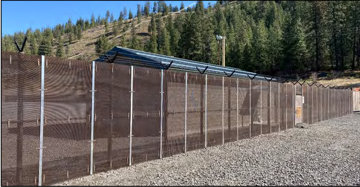
Figure 3 – Typical 9-foot Security Fence
