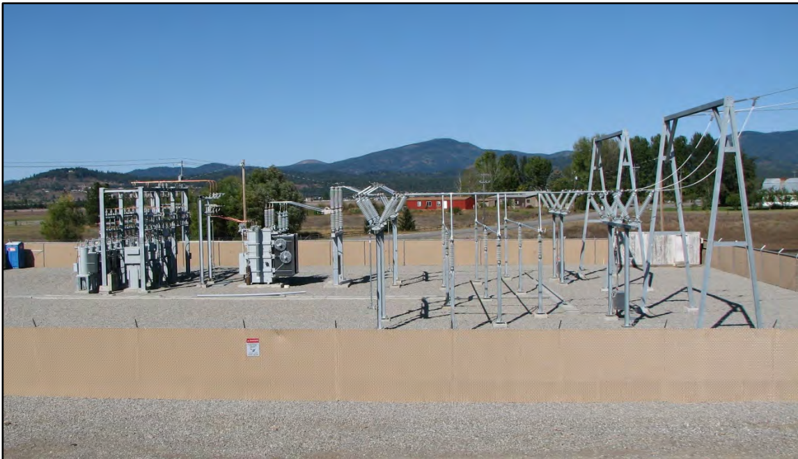
Figure 4 – Typical Distribution Substation
