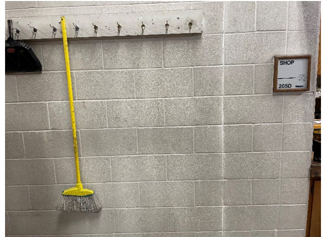
Photo 2. Close up view of CMU wall within Station 2 Engine Bay. Note the build-up of soot.
