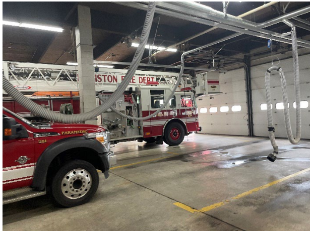
Photo 1. Overview of Station 1 Engine Bay. Light Soot build-up noted throughout bay.
