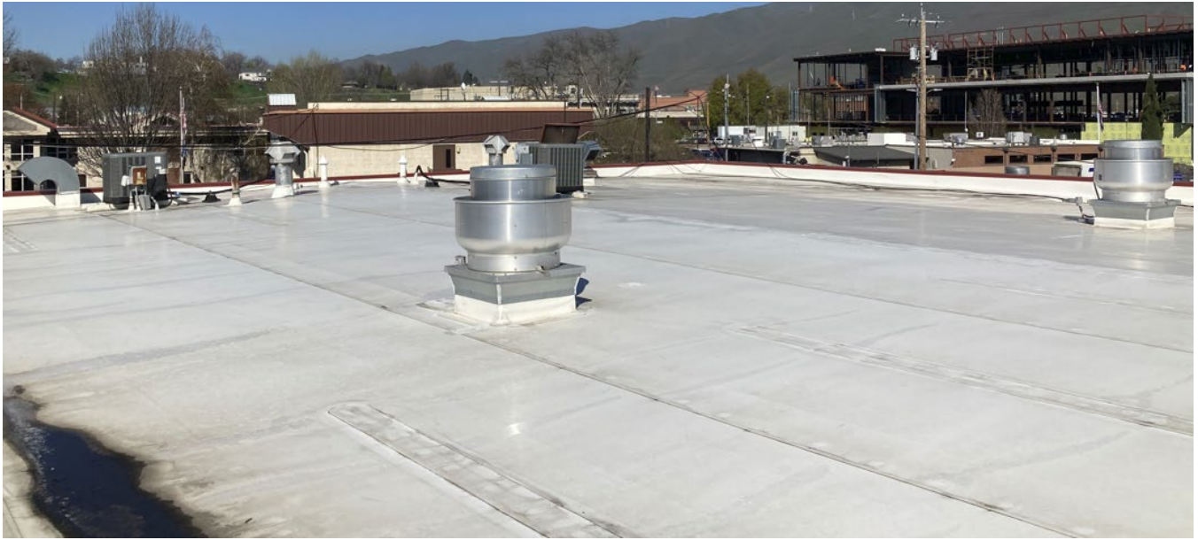
Existing Apparatus Bay General Exhaust Fans and Roof-Mounted Air Conditioners (beyond)
