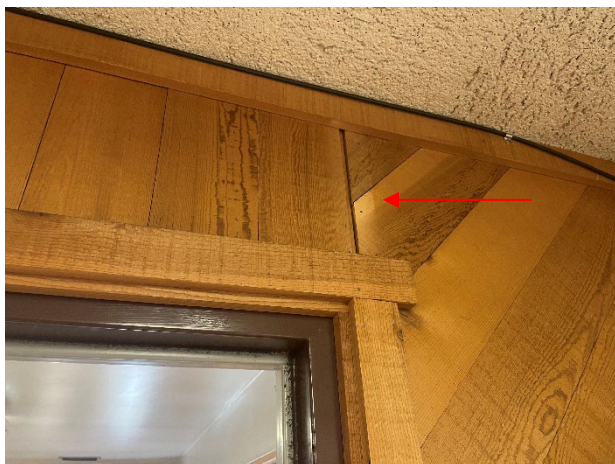
Photo 3. Close up view of porous building materials within Station 4. Note the staining where cedar trim was removed as indicated by the red arrow.
