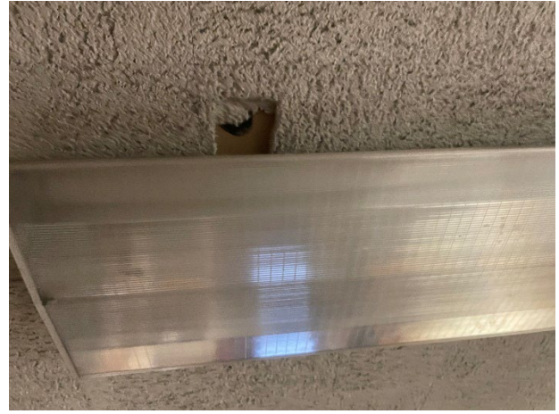
Photo 6. Close up view of soot-contaminated glued-on ceiling tile within Station 4.
