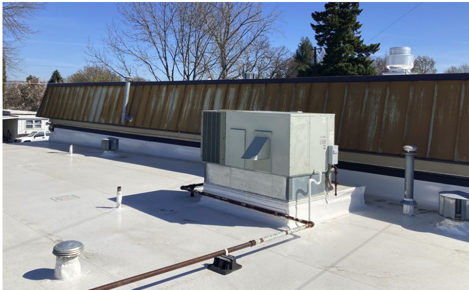
Existing Living Area Gas-Fired Packaged Roof-Top AC Unit
