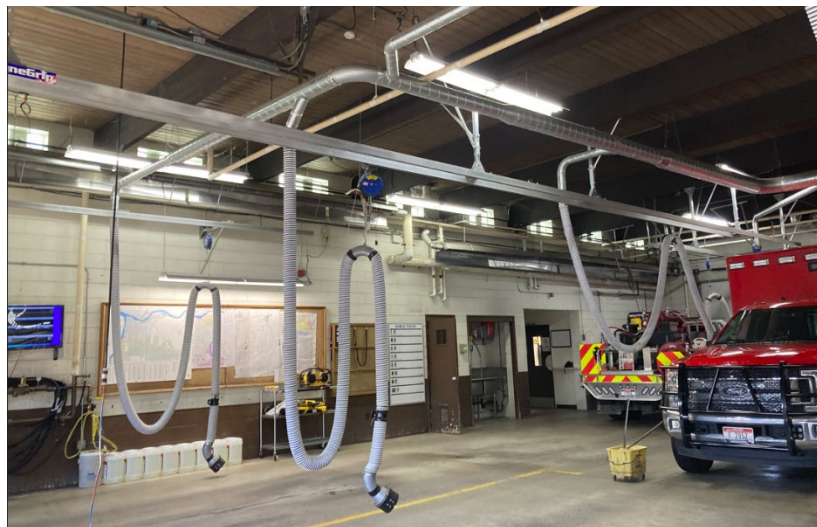
Existing Apparatus Bay Gas-Fired Radiant Tube Heaters and Tailpipe Exhaust System
