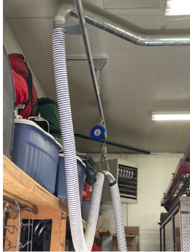
Existing Annex Gas-Fired Unit Heater Tailpipe Exhaust System
