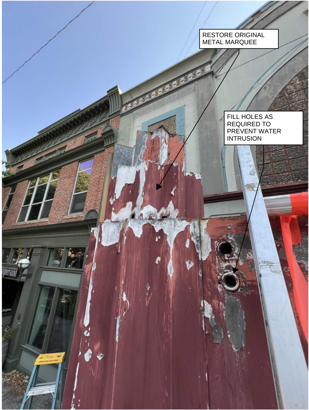
ORNAMENTAL FINIAL PEELING PAINT AT BOTH FINIALS
