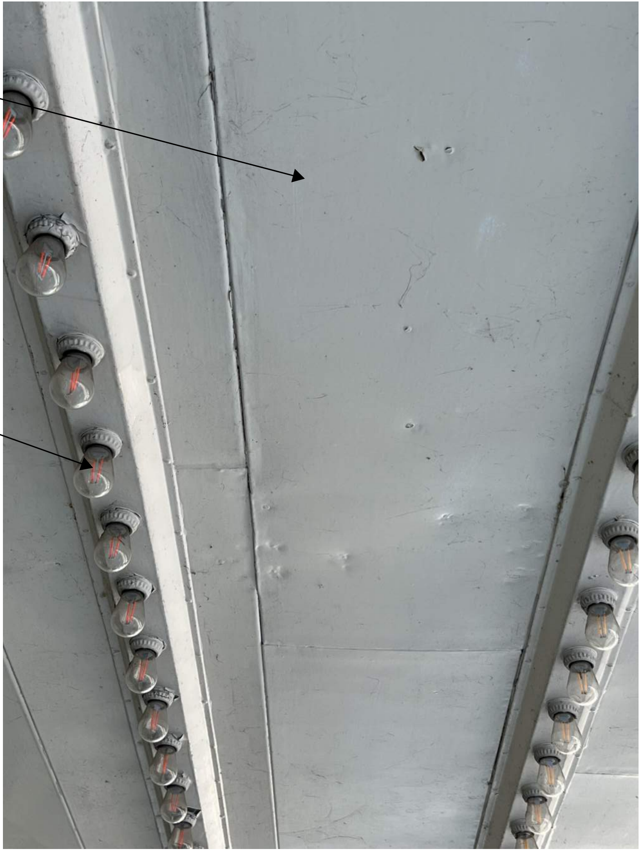
B.O. MARQUEE CONDITION LIGHTING AND METAL PANELING DIMPLING
