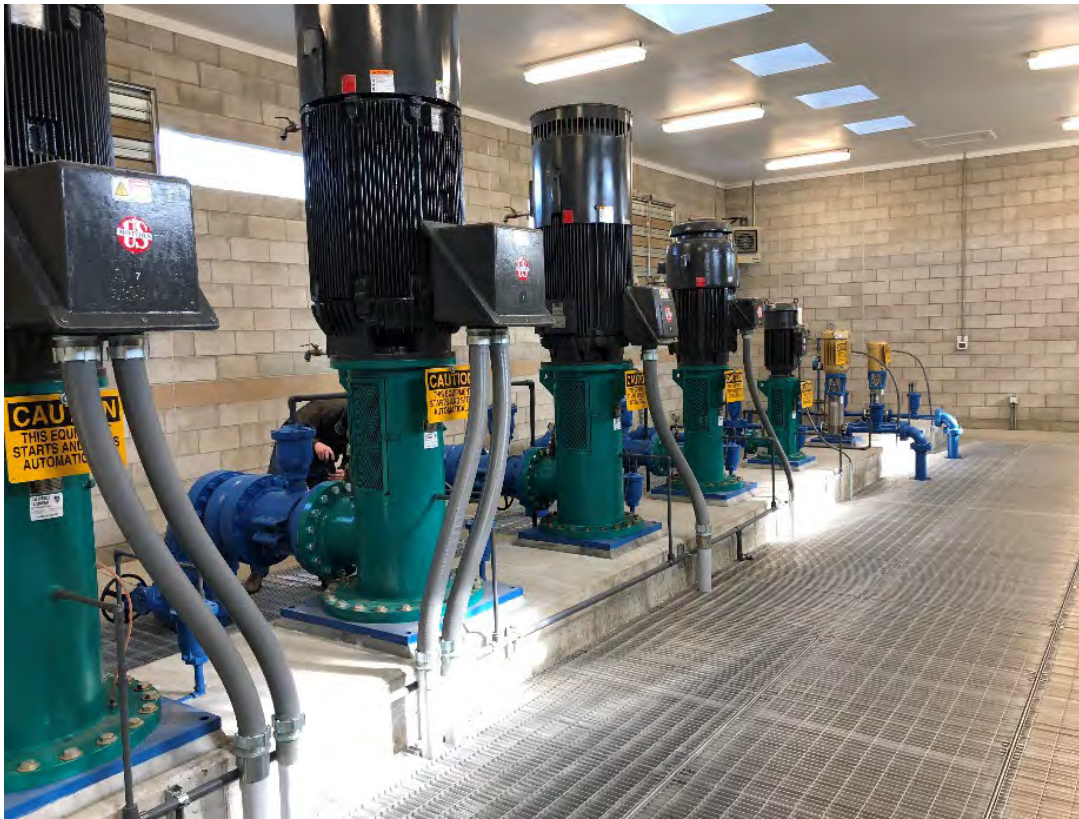
Photo 2-1: Southport Booster Station Interior
