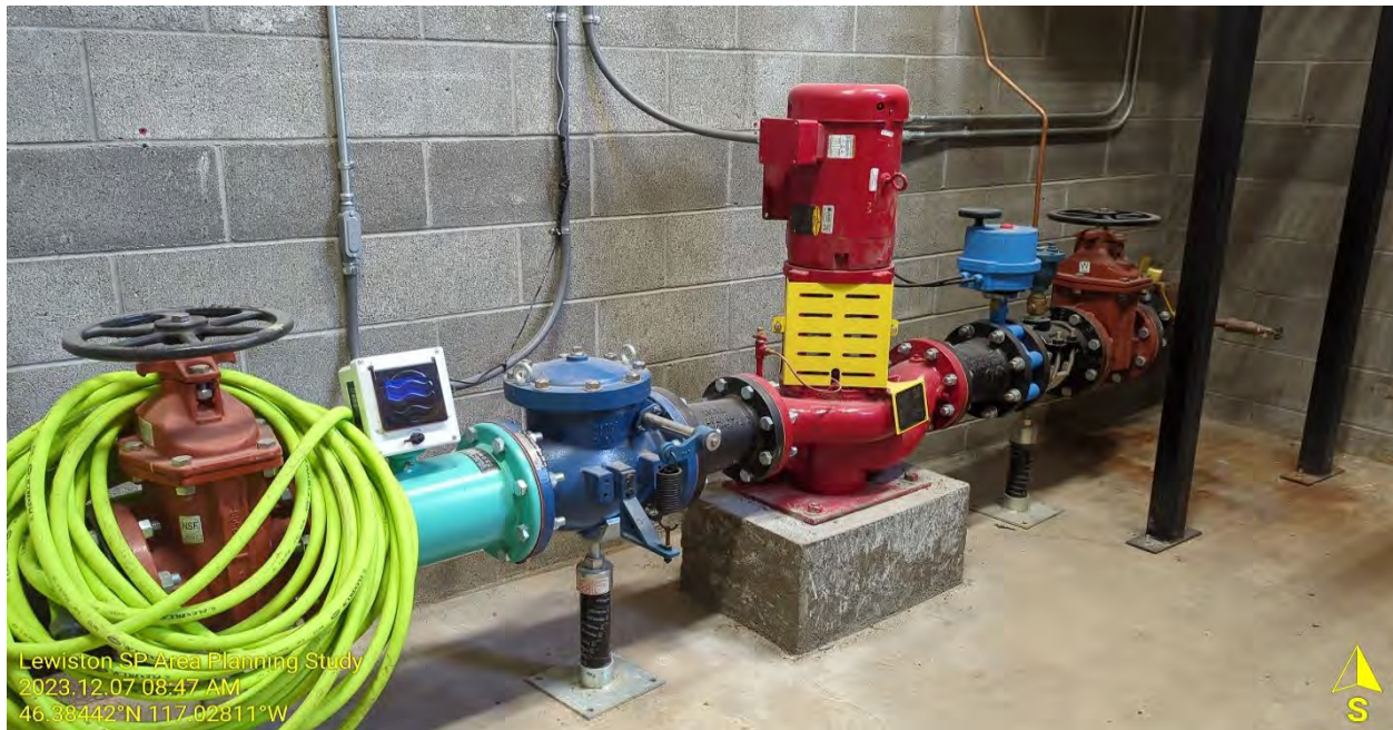
Photo 2-2: SW Small Booster Station Interior
