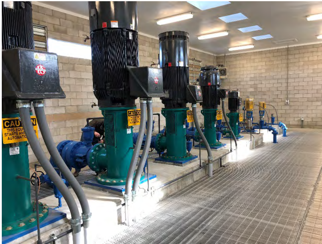
Photo 2-1: Southport Booster Station Interior
