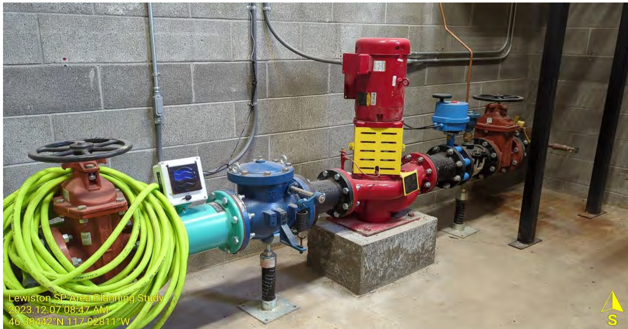
Photo 2-2: SW Small Booster Station Interior
