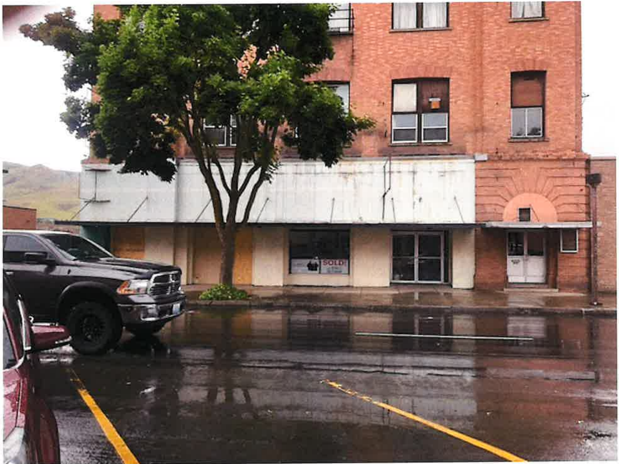
Front of building metal to be removed.
