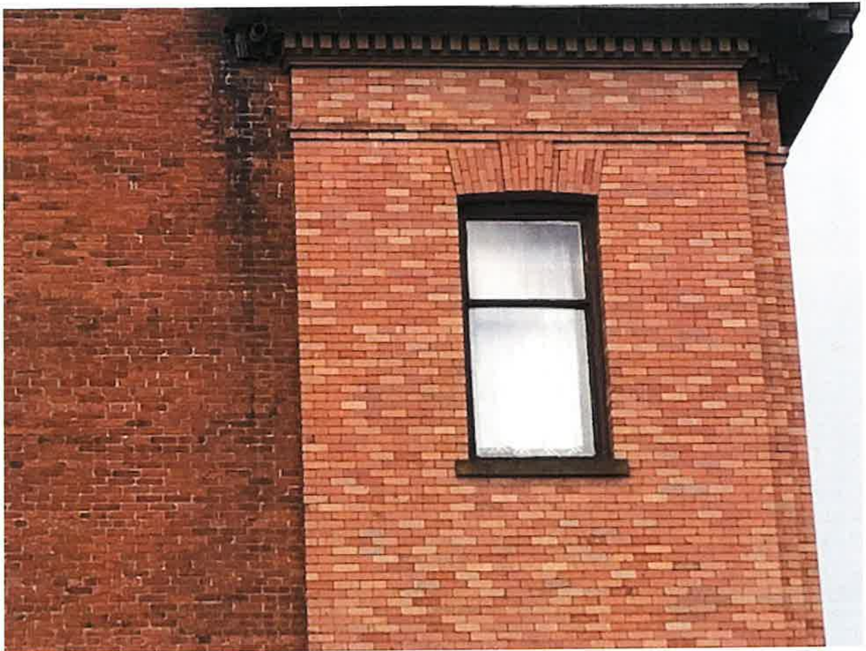
Example of window to be replaced
