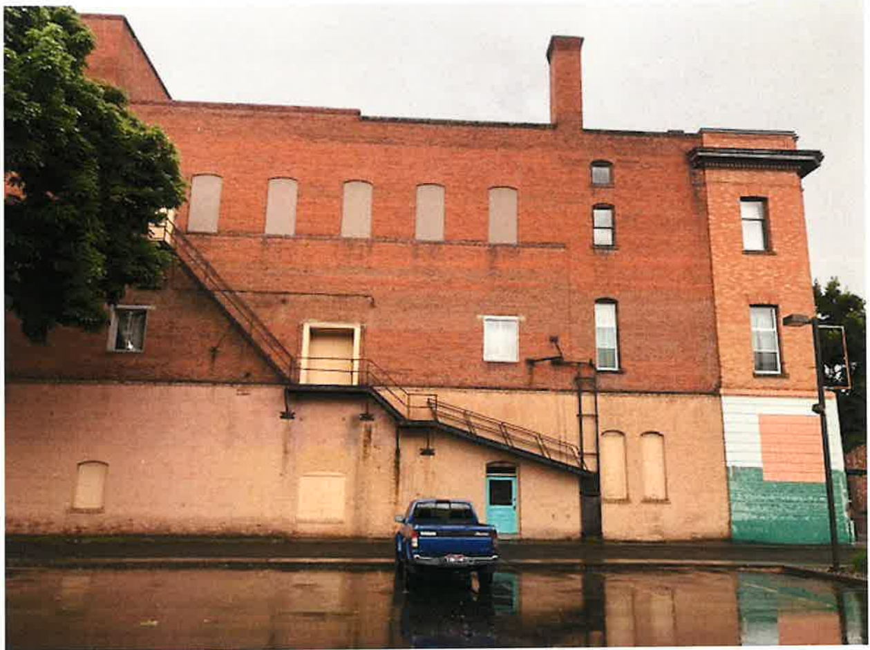
Paint to be removed on alley wall
